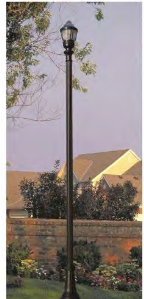
TYPICAL STREET LIGHTING
